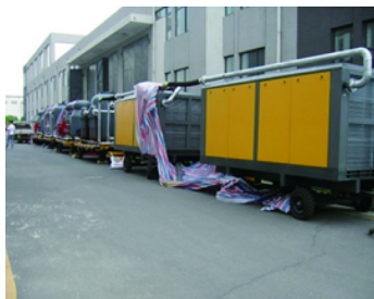
Fig. 70 Nitrogen generator at site test
