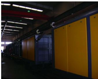
Fig. 69 Nitrogen generator after assembly
