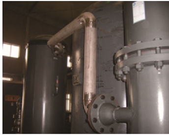
Fig. 67 Nitrogen generator in making
